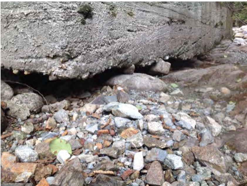
scour under right bank CIP - extends up to 800mm
