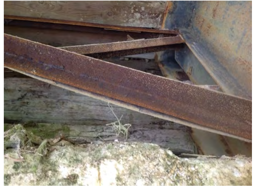
delamination of left bank diaphragm
